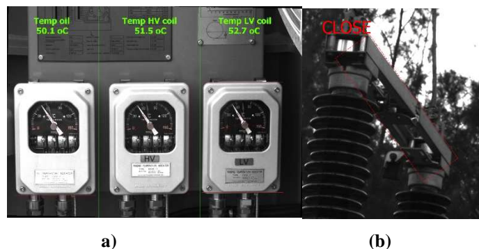
Figure 6: The Objects (a) The Meters of Transformer and (b) The Switch
